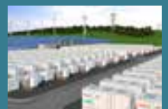
Renewable energy plant with stationary storage batteries
